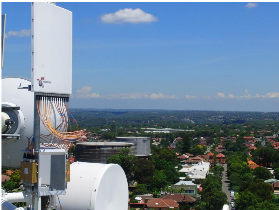
ETI's system facing south toward location of CPE
